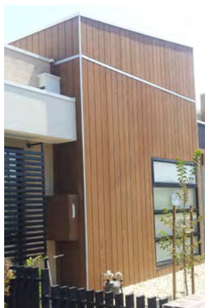
4 MONTHS: The board shows signs of lightening.
